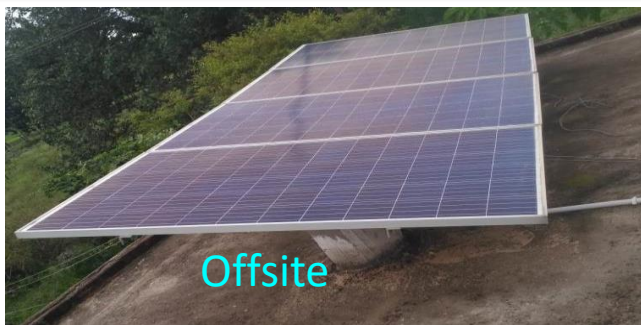
PV Solar Panel Installed at Intake Pump House
